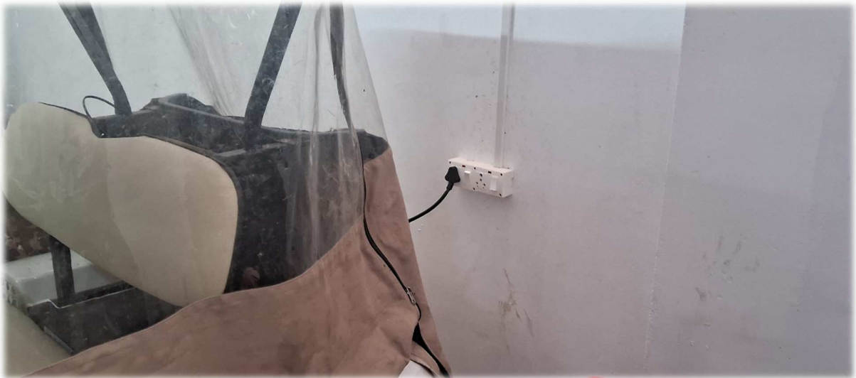
Electric vehicle charging station
