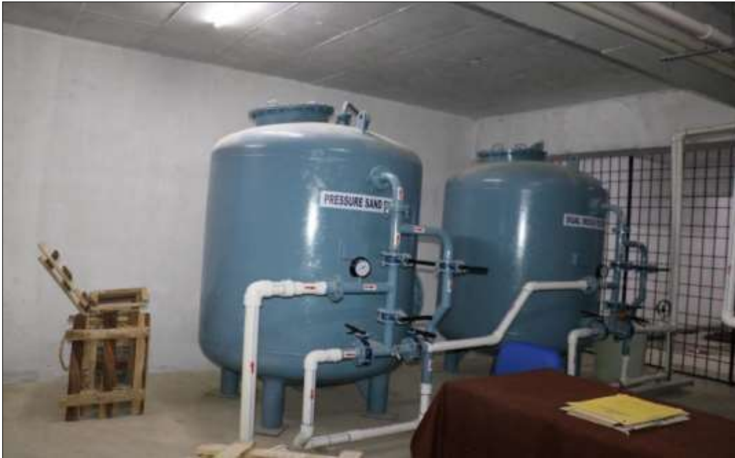
Figure 10: Pressure Sand Filter and Activated Carbon filter
