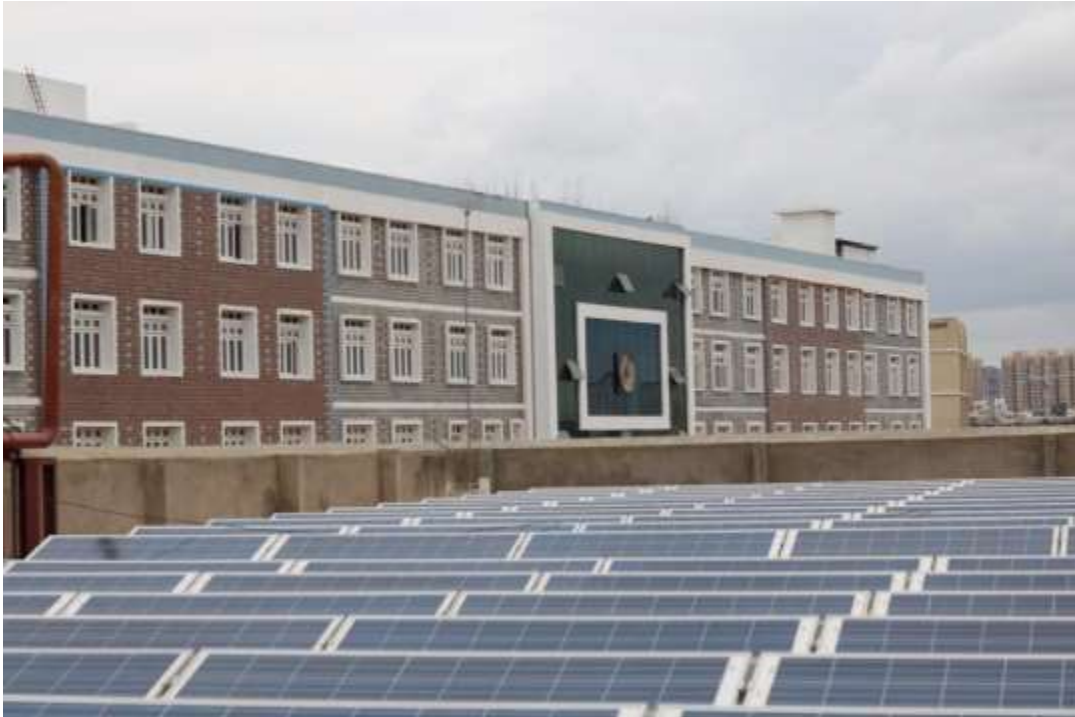
Figure 4 : Roof top SPV in campus
