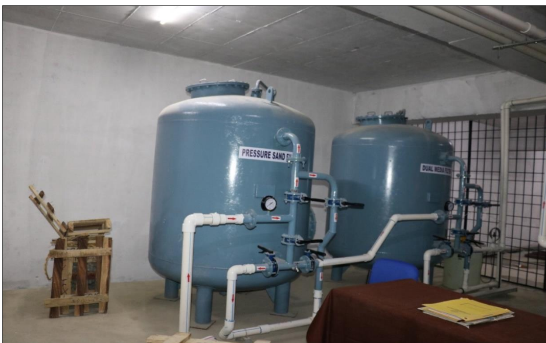
Figure 11: Pressure Sand Filter and Activated Carbon filter
