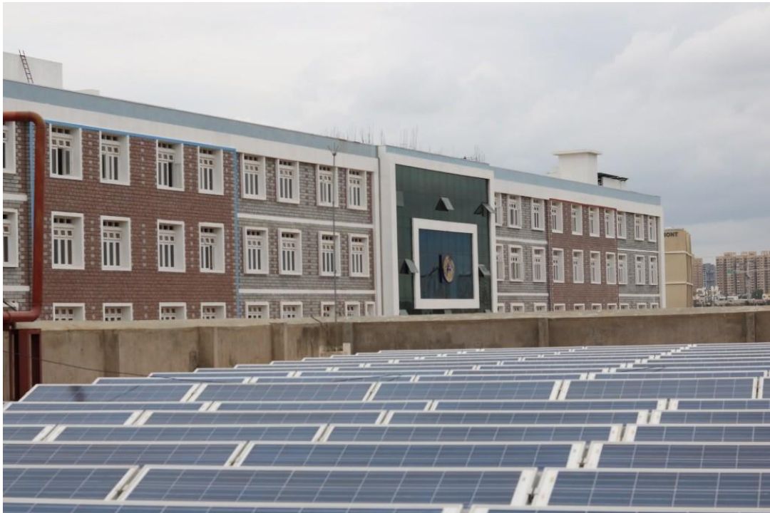
Figure 5: Roof top SPV in campus
