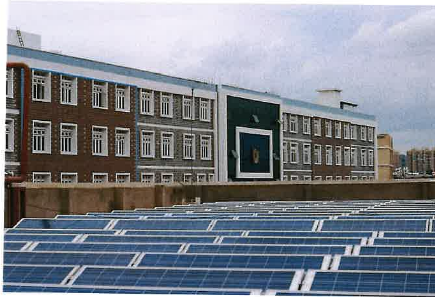
Figure 6: Roof top SPV in campus
