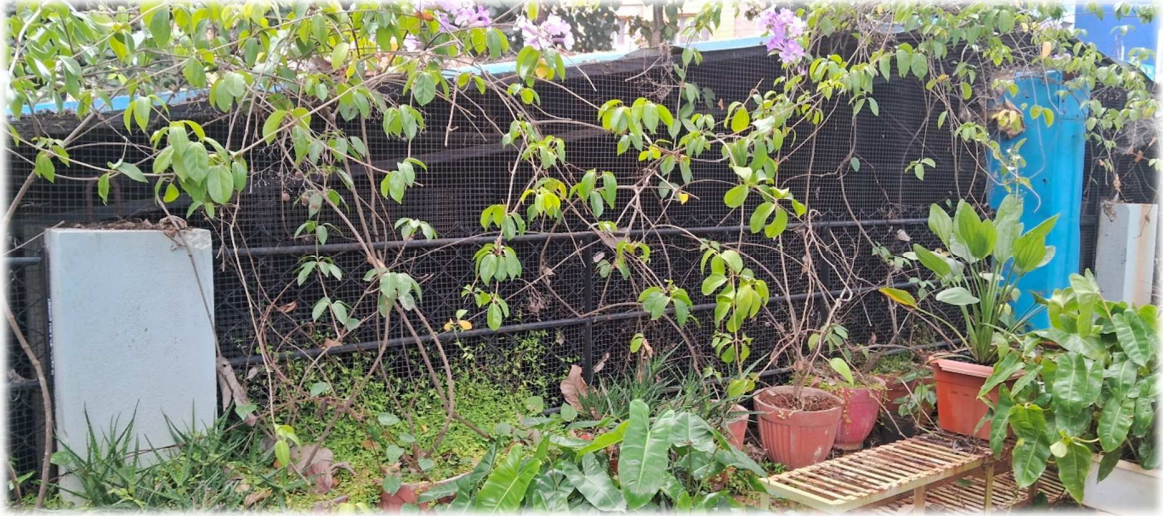
Rainwater storage tank
