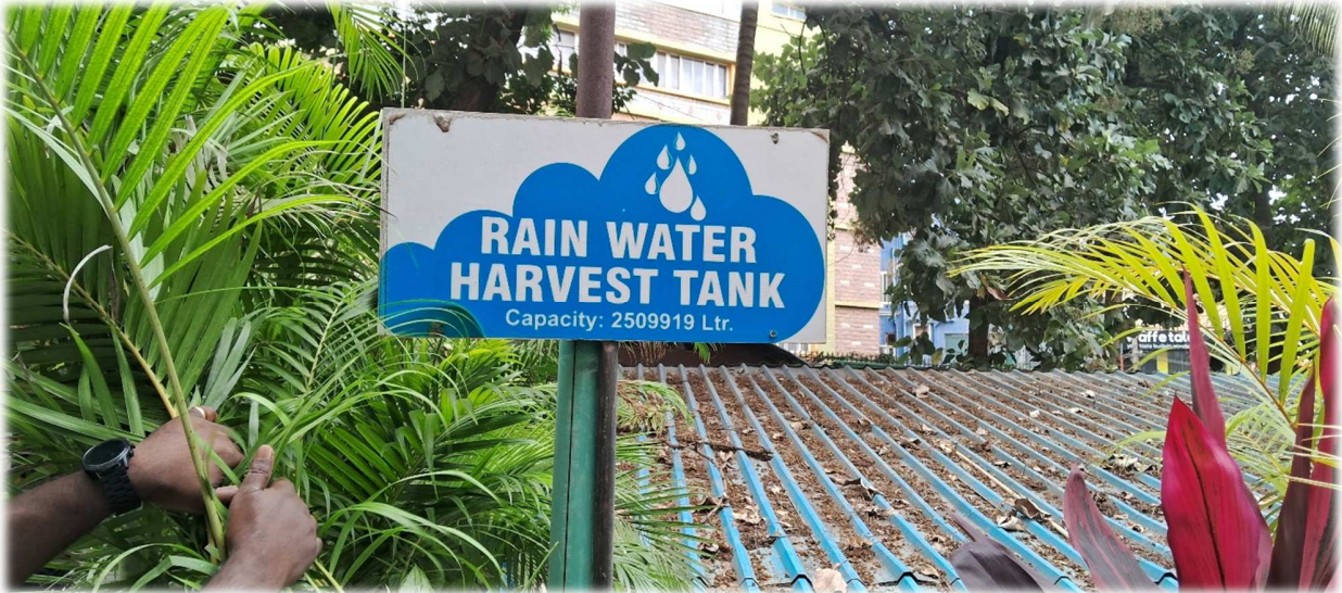
Rainwater storage tank
