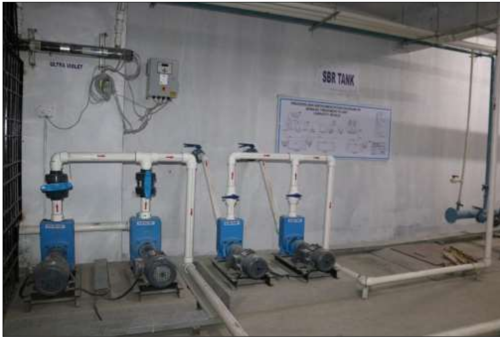
Figure 8: Sewage Treatment Plant (STP)
