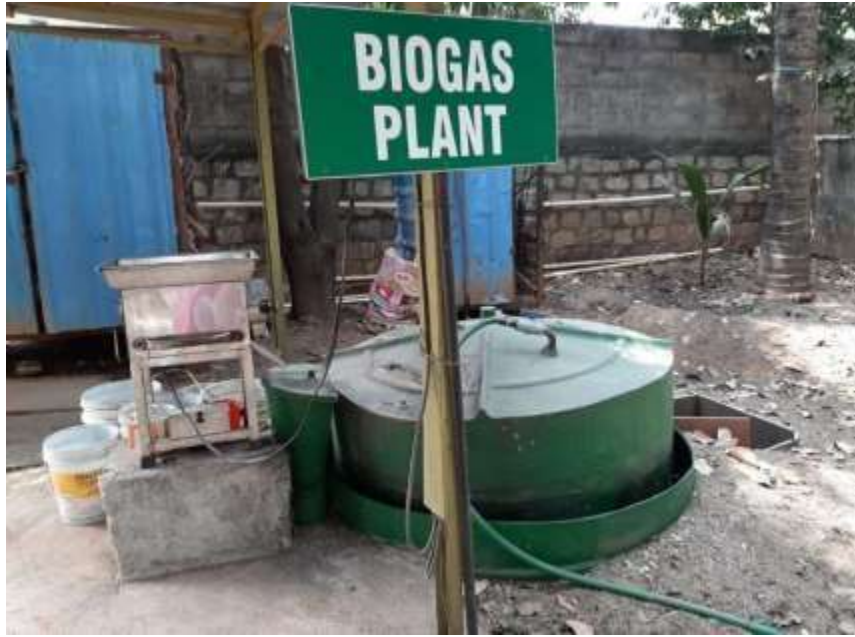
Figure 11: Biogas plant for Food waste
