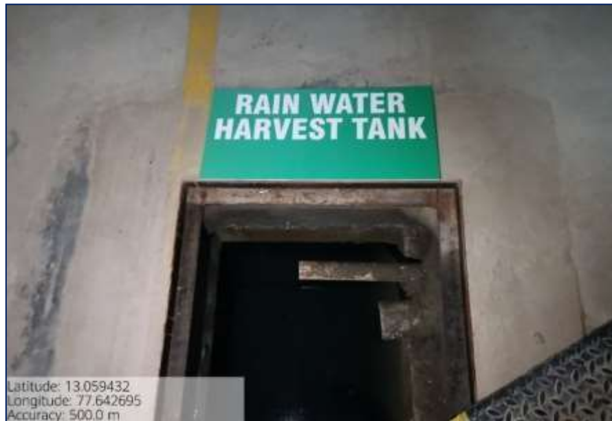
Figure 7: Rainwater harvesting tank near admin block
